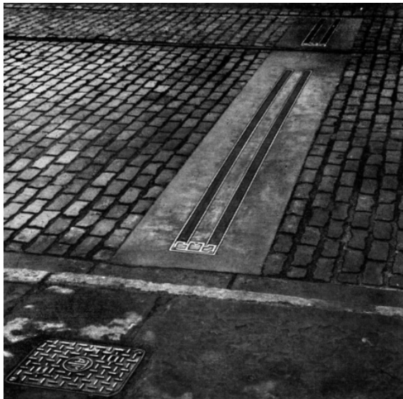
Figure 36: Pneumatic vehicle sensors, with pavement box housing control equipment, no date but before 1957 (Automatic Telephone & Electric Co. Ltd). 337
