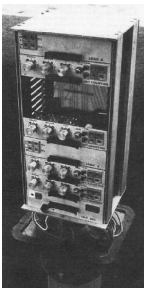
Figure 49: Queue-detector equipment in a roadside post-mounted box (Crown Copyright, Open Government License v3.0). 574
