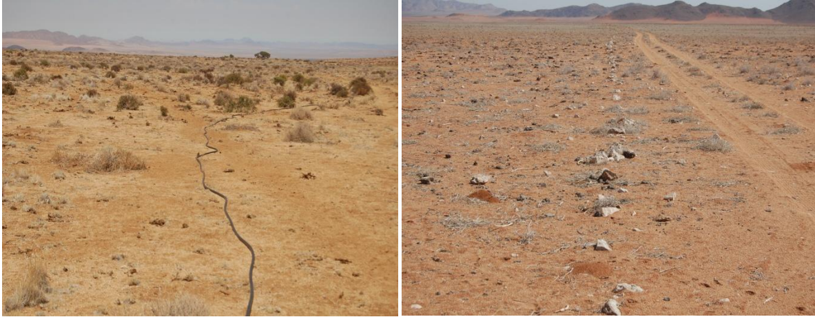
Figure 7.10: a (left) exposed water pipe on KAV, b (right) rocks on top of buried water pipe, Tsirub
