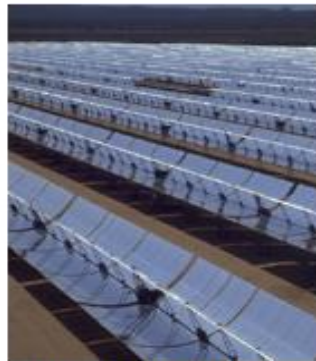
Concentrated Solar Power System
