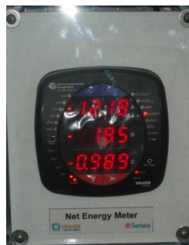
Plate 6: Net meter installed in a resident's home with renewable energy devices (Author 2011).
