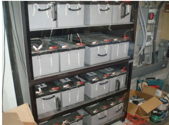
Plate 7: Bank of 16 batteries used for storage in a resident's home [RESI 1] with renewable energy devices installed (Author 2011).
